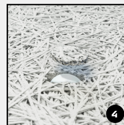
Place the drilled pieces of cement-bonded wood wool in the holes with sealant
